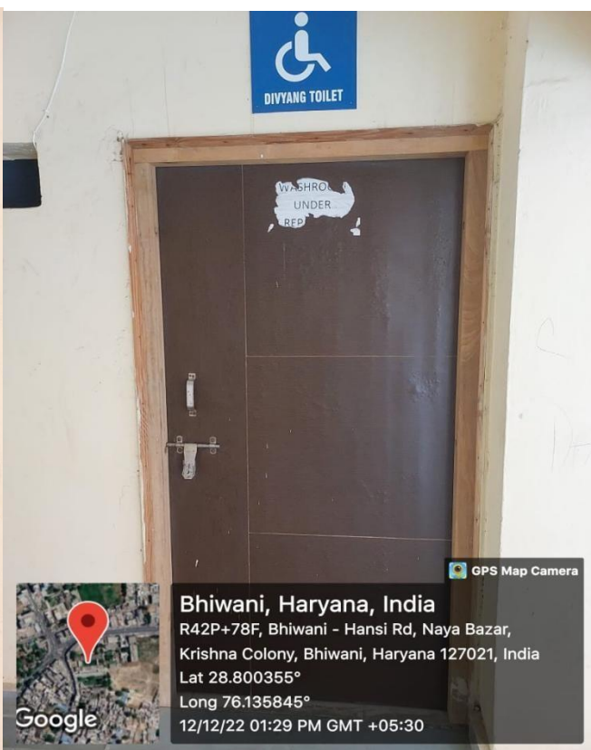
Toilet For Disabled
