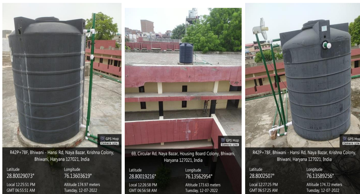
Fig: 6 Water Storage Tanks
