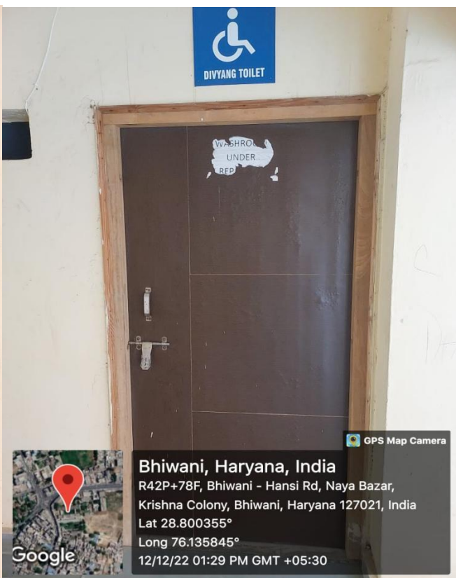
Toilet For Disabled
